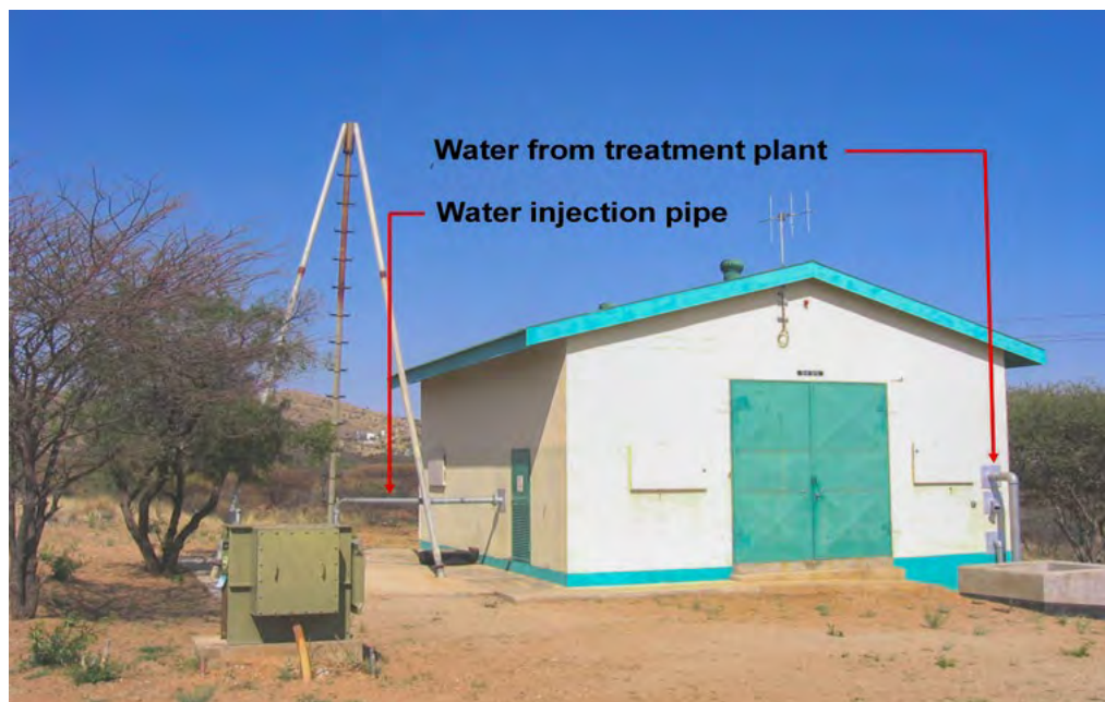
Figure 14: Artificial aquifer recharge station [Source: P Heyns]
