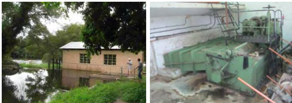
Figure 50: Andara power station, Okavango River (left) with 50kW generator [Source: P Heyns]
