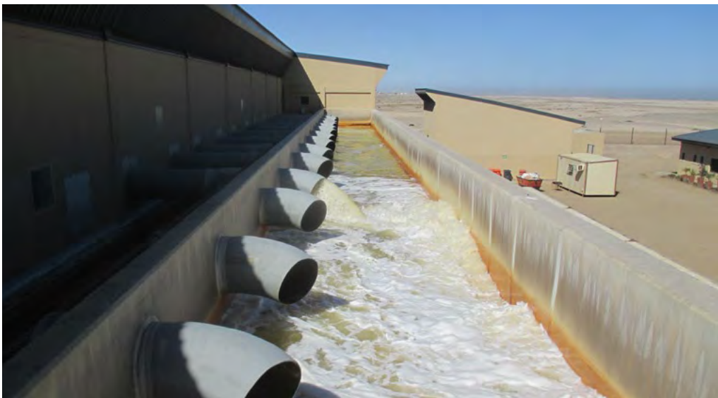
Figure 134: Effluent water from the Erongo Desalination Plant [Source: G Schneider]
